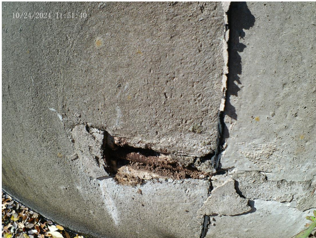
Figure 8: Exposed Rod at Expansion Joint
