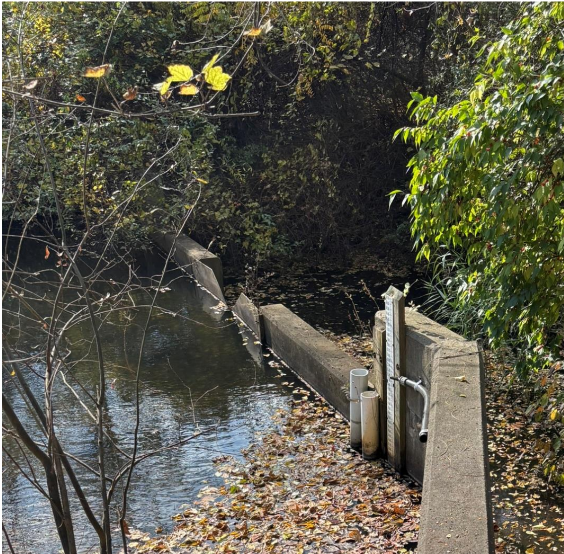
Figure 4: BMP #75 Installed Condition with V-Notch Weir
