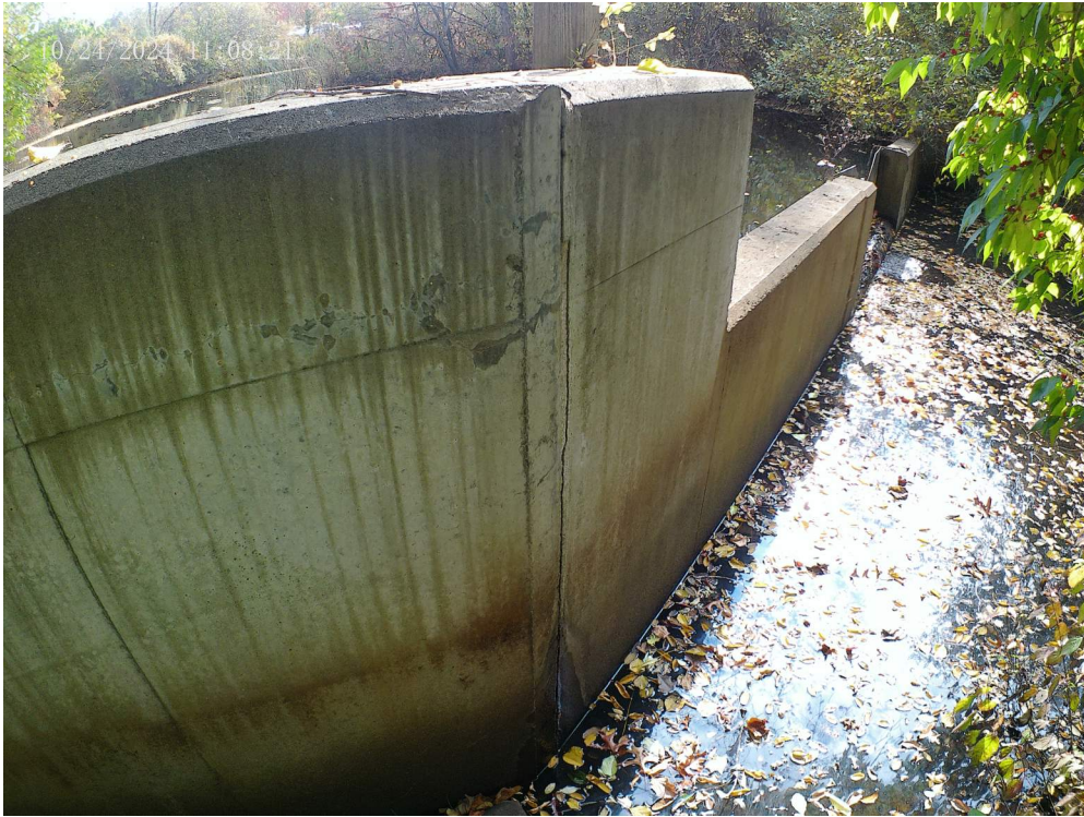
Photo 3. Outlet structure wall (downstream), some spalling at joints evident
