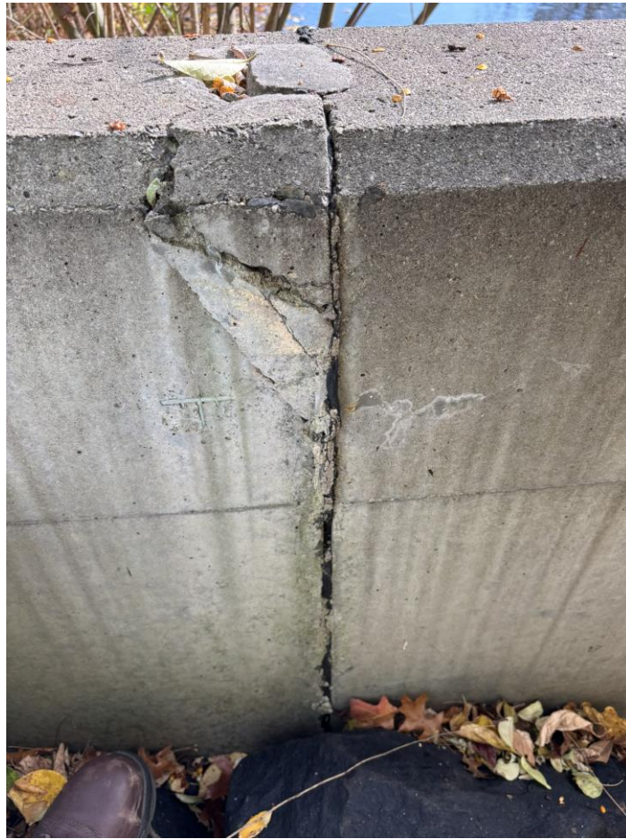
Figure 7: Spalling at Construction Joints
