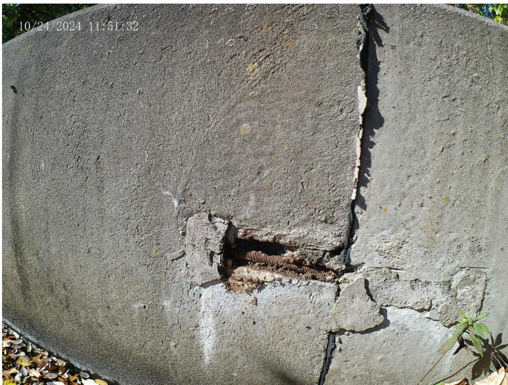
Photo 4. Outlet structure wall (upstream) showing exposure of dowel rod across expansion joint
